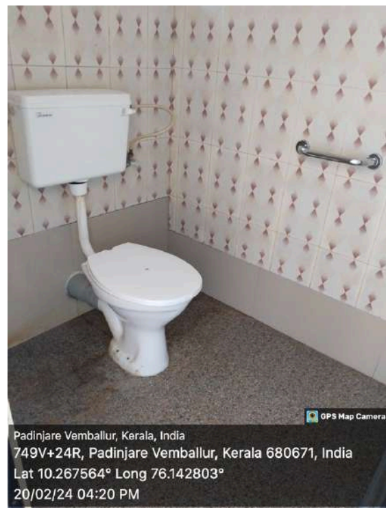
Washroom for differently Abled in the New Building
