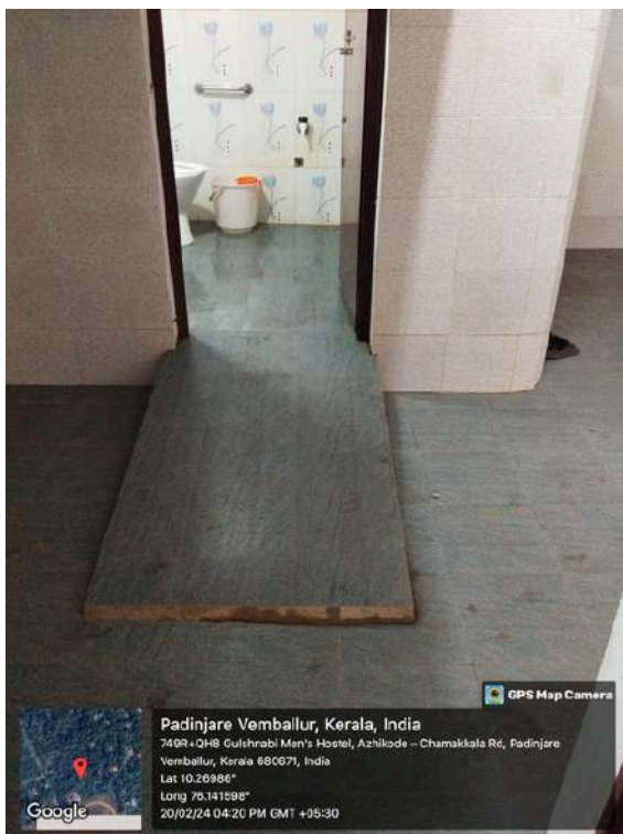
Washroom for Differently Abled in the Main block
