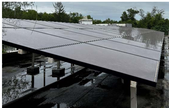
20kWp Solar Power plant
